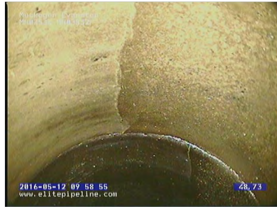
GM3702_bffedebf-8262-4dd8-8638-19abd94e99a5_20160512_100014_589.jpg, 00:05:58, 48.72 Crack Longitudinal at 10 o'clock, within 8 inch
