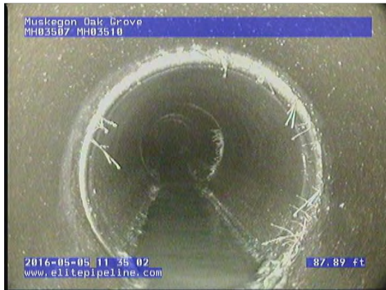
GM3676_29b5a4f6-782c-44a4-b604-e6dda5d2d56c_20160505_113639_283.jpg, 00:13:13, 87.89 Roots Fine Joint from 9 o'clock to 5 o'clock, within 8 inch
