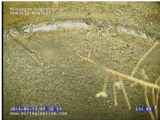
GM3701_62c62d3f-fa26-4182-aa9d-10e119c32db3_20160512_094018_482.jpg, 00:15:23, 233.10 Roots Fine Joint from 1 o'clock to 5 o'clock, within 8 inch
