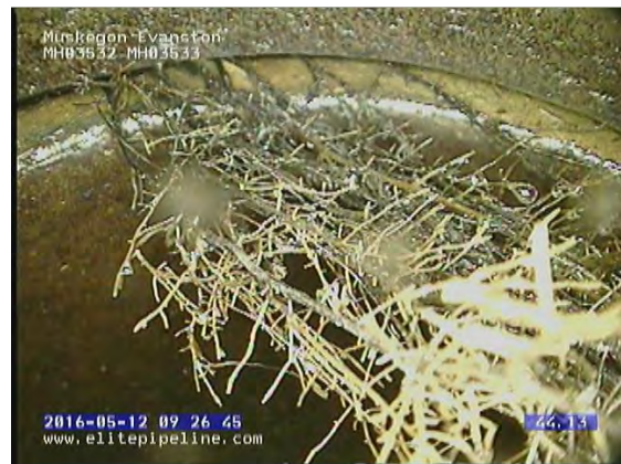
GM3701_62c62d3f-fa26-4182-aa9d-10e119c32db3_20160512_092804_746.jpg, 00:03:45, 43.20 Roots Fine Joint from 1 o'clock to 4 o'clock, within 8 inch
