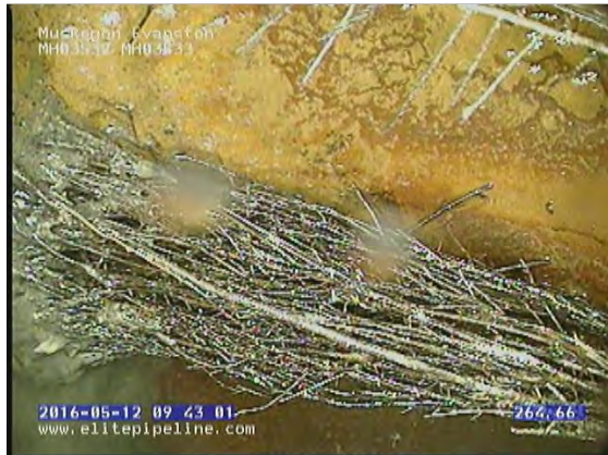
GM3701_62c62d3f-fa26-4182-aa9d-10e119c32db3_20160512_094420_095.jpg, 00:18:40, 263.46 Roots Fine Joint from 7 o'clock to 12 o'clock, within 8 inch
