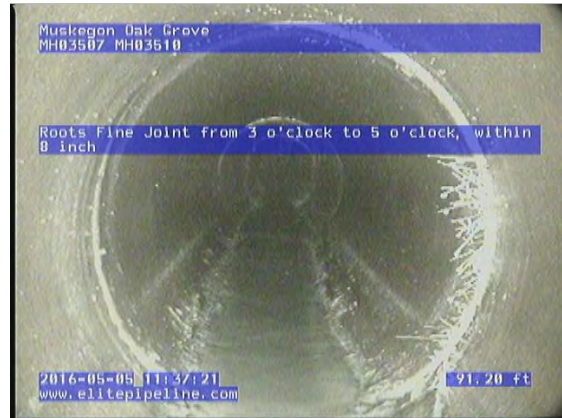
GM3676_29b5a4f6-782c-44a4-b604-e6dda5d2d56c_20160505_113858_220.jpg, 00:14:23, 91.19 Roots Fine Joint from 9 o'clock to 5 o'clock, Start, within 8 inch
