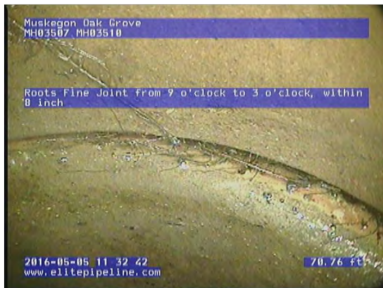
GM3676_29b5a4f6-782c-44a4-b604-e6dda5d2d56c_20160505_113419_024.jpg, 00:11:13, 70.76 Roots Fine Joint from 9 o'clock to 3 o'clock, within 8 inch
