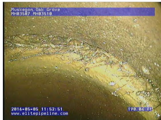
GM3676_29b5a4f6-782c-44a4-b604-e6dda5d2d56c_20160505_115428_369.jpg, 00:26:35, 189.32 Infiltration Dripper at 10 o'clock, within 8 inch
