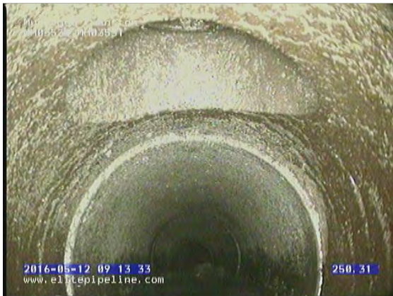
GM3700_d760bc2d-7738-420b-a21c-0e3d9fae79d8_20160512_091452_627.jpg, 00:16:30, 250.29 Tap Factory Made at 12 o'clock, 6inch dim, within 8 inch
