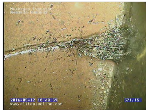
GM3702_bffedebf-8262-4dd8-8638-19abd94e99a5_20160512_104218_547.jpg, 00:37:33, 370.26 Roots Fine Joint from 8 o'clock to 4 o'clock, within 8 inch
