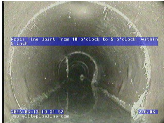
GM3702_bffedebf-8262-4dd8-8638-19abd94e99a5_20160512_102315_934.jpg, 00:23:57, 270.04 Roots Fine Joint from 10 o'clock to 5 o'clock, within 8 inch
