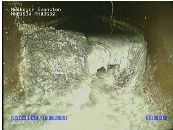
GM3702_bffedebf-8262-4dd8-8638-19abd94e99a5_20160512_103710_711.jpg, 00:33:56, 331.81 Deposits Settled Other, 20% of cross sectional area from 4 o'clock to 8 o'clock, Debris
