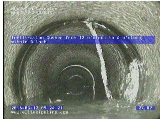
GM3701_62c62d3f-fa26-4182-aa9d-10e119c32db3_20160512_092540_357.jpg, 00:01:55, 27.89 Infiltration Gusher from 12 o'clock to 4 o'clock, within 8 inch
