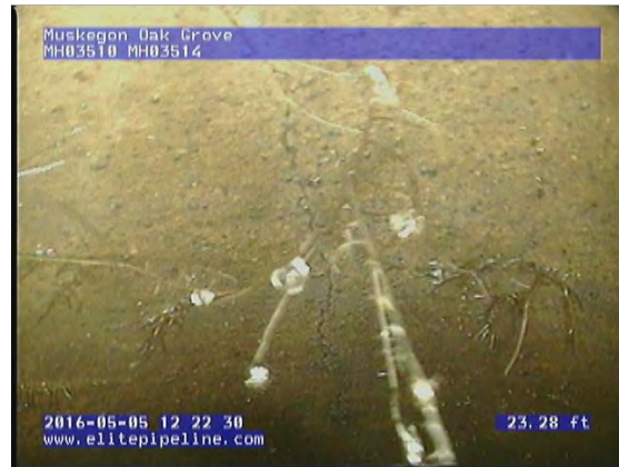
GM3683_ed2824f5-d3e3-4757-88d6-d4208adc31ee_20160505_122406_744.jpg, 00:04:13, 23.27 Crack Longitudinal at 12 o'clock, within 8 inch
