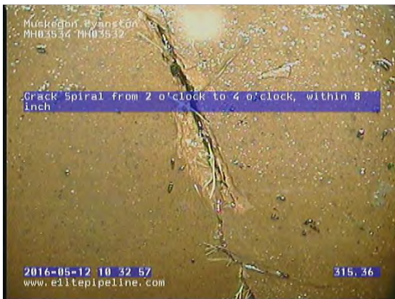
GM3702_bffedebf-8262-4dd8-8638-19abd94e99a5_20160512_103416_302.jpg, 00:31:47, 315.36 Crack Spiral from 2 o'clock to 4 o'clock, within 8 inch
