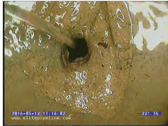
GM3702_bffedebf-8262-4dd8-8638-19abd94e99a5_20160512_111721_431.jpg, 00:40:00, 221.35 General Observation, This hole is at MH03534, verified from the top outside the pipe.
