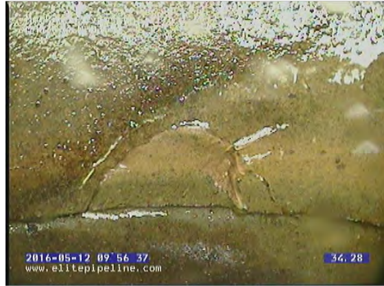
GM3702_bffedebf-8262-4dd8-8638-19abd94e99a5_20160512_095756_416.jpg, 00:03:59, 33.44 Infiltration Runner at 2 o'clock, within 8 inch
