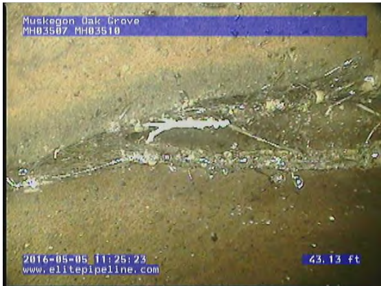
GM3676_29b5a4f6-782c-44a4-b604-e6dda5d2d56c_20160505_112700_276.jpg, 00:06:26, 42.24 Roots Fine Joint at 2 o'clock, within 8 inch
