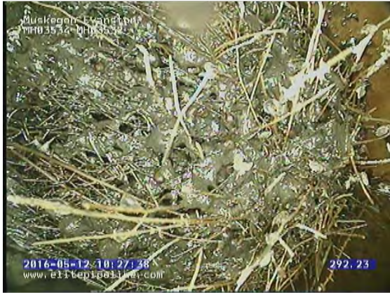
GM3702_bffedebf-8262-4dd8-8638-19abd94e99a5_20160512_102857_697.jpg, 00:27:24, 291.13 Roots Medium Joint from 7 o'clock to 9 o'clock, 10% lost, within 8 inch
