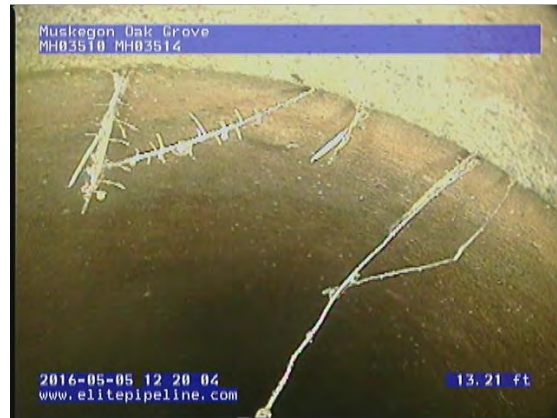
GM3683_ed2824f5-d3e3-4757-88d6-d4208adc31ee_20160505_122141_153.jpg,00:02:11,12.47 Roots Fine Joint from 11 o'clock to 2 o'clock, within 8 inch
