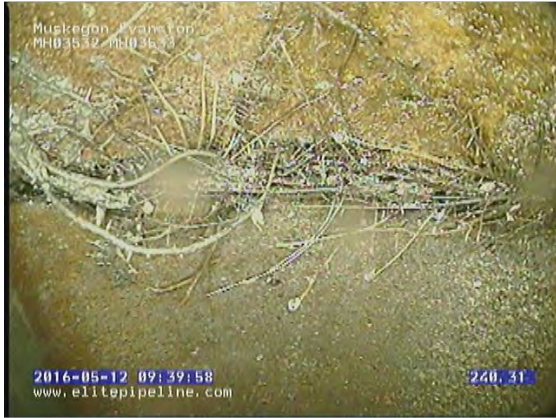
GM3701_62c62d3f-fa26-4182-aa9d-10e119c32db3_20160512_094117_401.jpg, 00:16:08, 239.43 Roots Fine Joint from 7 o'clock to 10 o'clock, within 8 inch
