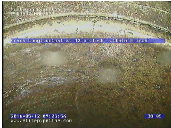
GM3701_62c62d3f-fa26-4182-aa9d-10e119c32db3_20160512_092713_281.jpg, 00:03:15, 38.04 Crack Longitudinal at 12 o'clock, within 8 inch
