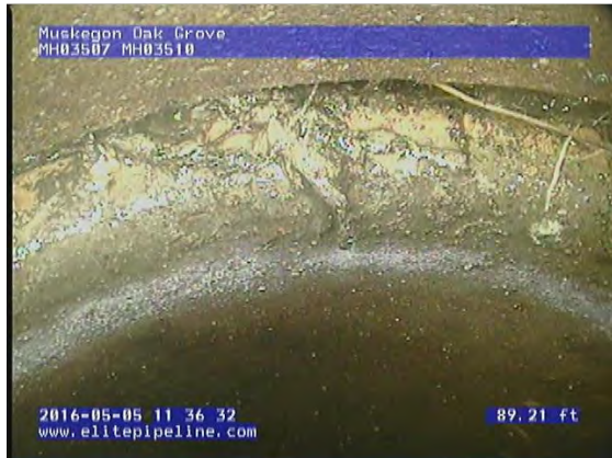
GM3676_29b5a4f6-782c-44a4-b604-e6dda5d2d56c_20160505_113809_419.jpg, 00:13:22, 87.89 Infiltration Dripper at 12 o'clock, within 8 inch
