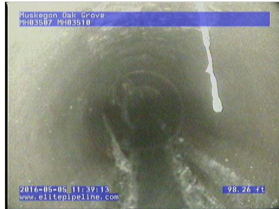
GM3676_29b5a4f6-782c-44a4-b604-e6dda5d2d56c_20160505_114049_830.jpg, 00:15:51, 97.59 Infiltration Dripper at 12 o'clock, within 8 inch
