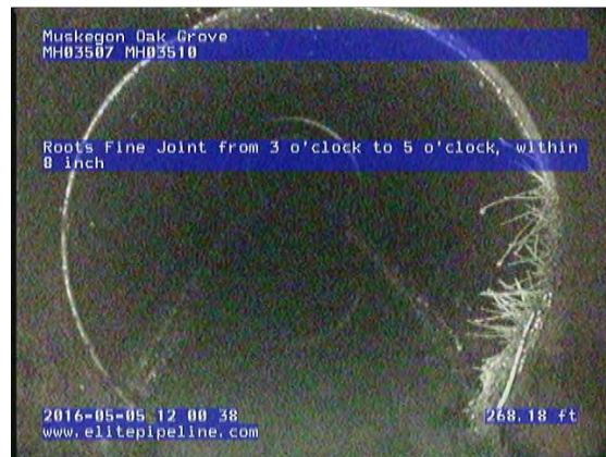
GM3676_29b5a4f6-782c-44a4-b604-e6dda5d2d56c_20160505_120215_554.jpg, 00:33:56, 268.17 Roots Fine Joint from 3 o'clock to 5 o'clock, within 8 inch
