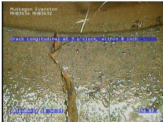
GM3702_bffedebf-8262-4dd8-8638-19abd94e99a5_20160512_103530_888.jpg, 00:32:39, 316.87 Crack Longitudinal at 3 o'clock, within 8 inch
