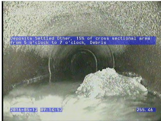
GM3700_d760bc2d-7738-420b-a21c-0e3d9fae79d8_20160512_091611_340.jpg, 00:17:22, 255.46 Deposits Settled Other, 15% of cross sectional area from 5 o'clock to 7 o'clock, Debris
