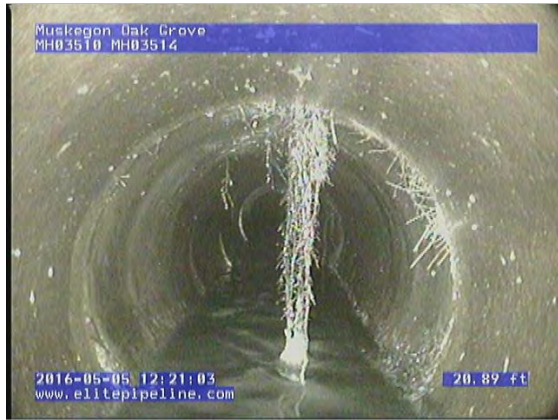
GM3683_ed2824f5-d3e3-4757-88d6-d4208adc31ee_20160505_122240_438.jpg, 00:03:10, 20.89 Roots Fine Joint from 10 o'clock to 3 o'clock, within 8 inch
