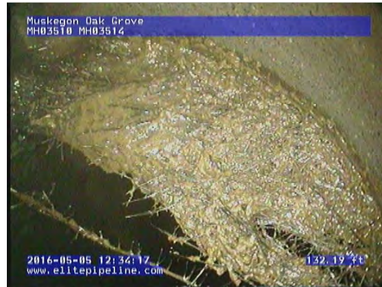
GM3683_ed2824f5-d3e3-4757-88d6-d4208adc31ee_20160505_123554_462.jpg, 00:13:49, 131.34 Roots Medium Joint from 7 o'clock to 3 o'clock, 20% lost, within 8 inch
