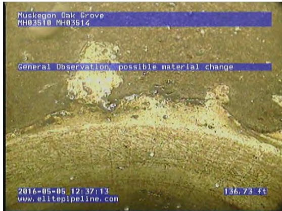
GM3683_ed2824f5-d3e3-4757-88d6-d4208adc31ee_20160505_123850_542.jpg, 00:15:52, 136.72 General Observation, possible material change
