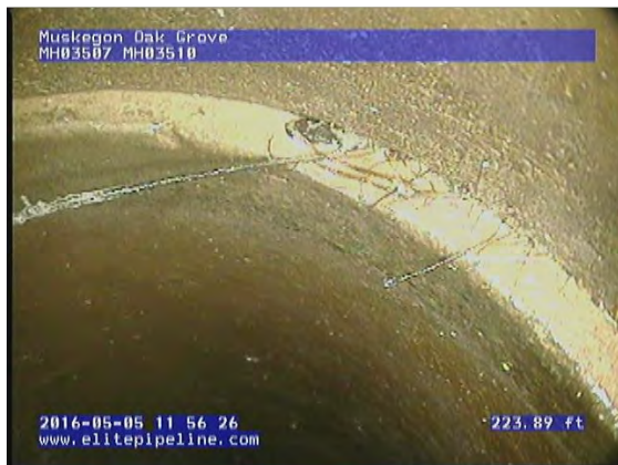
GM3676_29b5a4f6-782c-44a4-b604-e6dda5d2d56c_20160505_115802_730.jpg, 00:29:53, 223.07 Roots Fine Joint from 10 o'clock to 2 o'clock, within 8 inch
