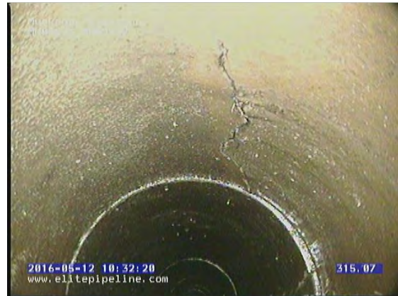
GM3702_bffedebf-8262-4dd8-8638-19abd94e99a5_20160512_103338_965.jpg, 00:31:09, 315.07 Crack Longitudinal at 12 o'clock, within 8 inch
