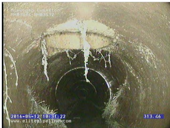
GM3702_bffedebf-8262-4dd8-8638-19abd94e99a5_20160512_103241_628.jpg, 00:30:29, 313.46 Tap Break-In at 12 o'clock, 6inch dim
