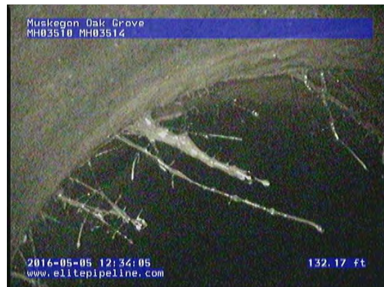
GM3683_ed2824f5-d3e3-4757-88d6-d4208adc31ee_20160505_123542_297.jpg, 00:13:55, 131.36 Infiltration Dripper at 1 o'clock, within 8 inch
