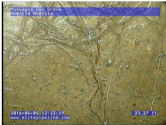
GM3683_ed2824f5-d3e3-4757-88d6-d4208adc31ee_20160505_122356_269.jpg, 00:04:13, 23.27 Crack Longitudinal at 12 o'clock, within 8 inch
