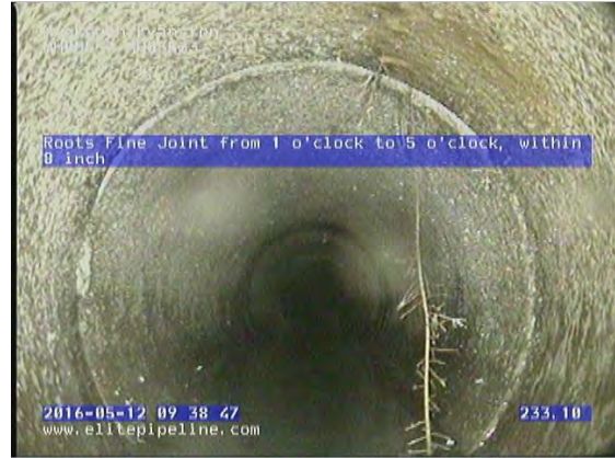
GM3701_62c62d3f-fa26-4182-aa9d-10e119c32db3_20160512_094006_610.jpg, 00:15:23, 233.10 Roots Fine Joint from 1 o'clock to 5 o'clock, within 8 inch
