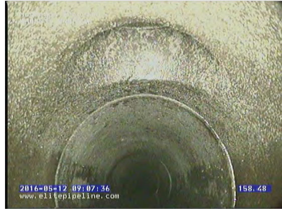
GM3700_d760bc2d-7738-420b-a21c-0e3d9fae79d8_20160512_090855_710.jpg, 00:11:02, 158.48 Tap Factory Made at 12 o'clock, 6inch dim, within 8 inch
