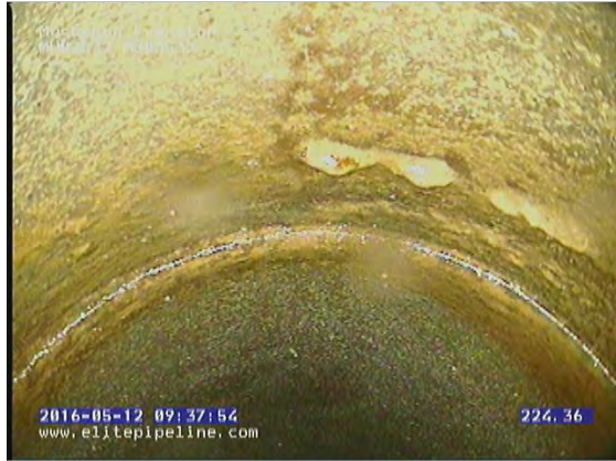
GM3701_62c62d3f-fa26-4182-aa9d-10e119c32db3_20160512_093913_327.jpg, 00:14:41, 224.36 Infiltration Dripper at 12 o'clock, within 8 inch
