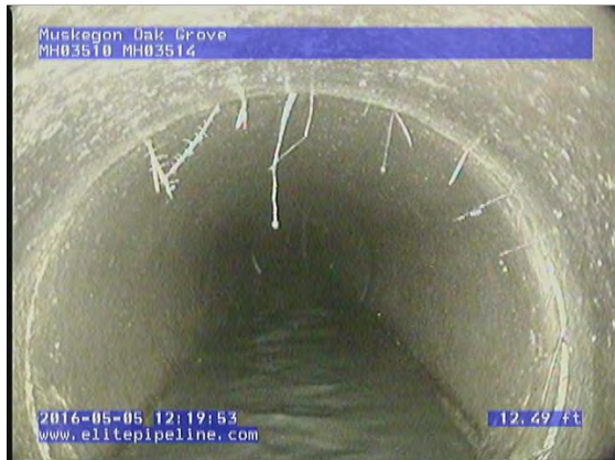
GM3683_ed2824f5-d3e3-4757-88d6-d4208adc31ee_20160505_122130_003.jpg,00:02:11,12.47 Roots Fine Joint from 11 o'clock to 2 o'clock, within 8 inch
