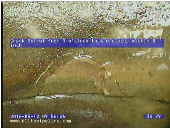
GM3702_bffedebf-8262-4dd8-8638-19abd94e99a5_20160512_095815_682.jpg, 00:04:25, 34.28 Crack Spiral from 3 o'clock to 4 o'clock, within 8 inch
