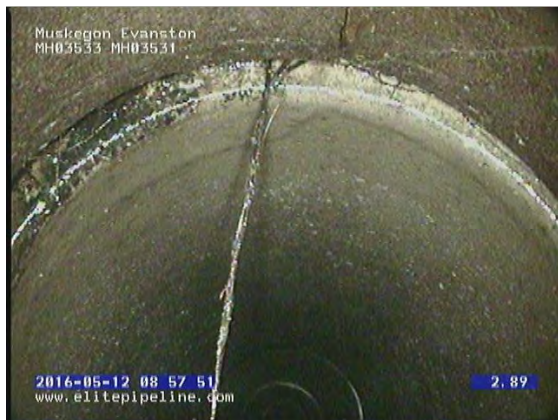
GM3700_d760bc2d-7738-420b-a21c-0e3d9fae79d8_20160512_085910_343.jpg, 00:03:29, 2.89 Roots Fine Joint at 12 o'clock, within 8 inch
