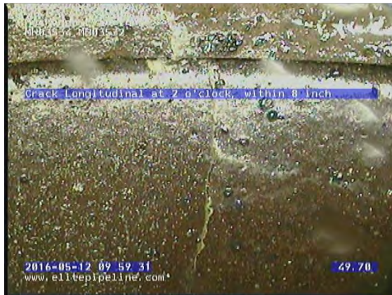
GM3702_bffedebf-8262-4dd8-8638-19abd94e99a5_20160512_100050_142.jpg, 00:06:32, 49.70 Crack Longitudinal at 2 o'clock, within 8 inch
