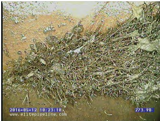
GM3702_bffedebf-8262-4dd8-8638-19abd94e99a5_20160512_102429_325.jpg, 00:24:38, 273.04 Roots Fine Joint from 10 o'clock to 5 o'clock, within 8 inch
