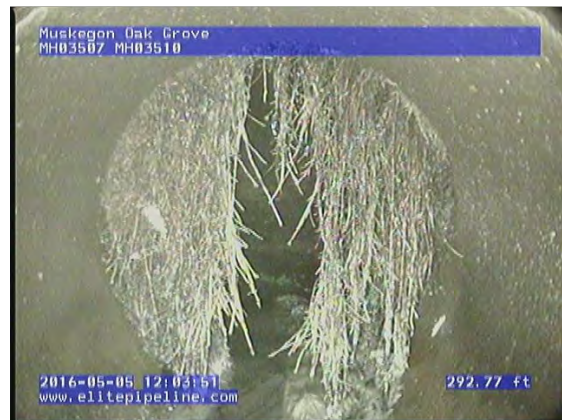
GM3676_29b5a4f6-782c-44a4-b604-e6dda5d2d56c_20160505_120527_848.jpg, 00:36:28, 292.77 Roots Ball Joint from 7 o'clock to 5 o'clock, 75% lost, within 8 inch
