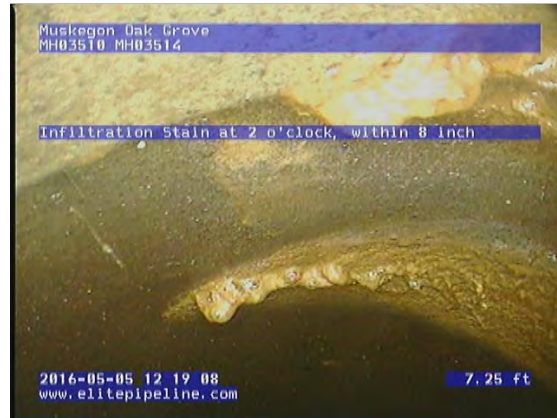
GM3683_ed2824f5-d3e3-4757-88d6-d4208adc31ee_20160505_122045_186.jpg,00:01:39,7.24 Infiltration Stain at 2 o'clock, within 8 inch
