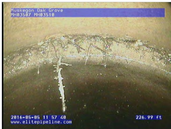
GM3676_29b5a4f6-782c-44a4-b604-e6dda5d2d56c_20160505_115916_947.jpg, 00:30:43, 226.34 Roots Fine Joint from 9 o'clock to 12 o'clock, within 8 inch
