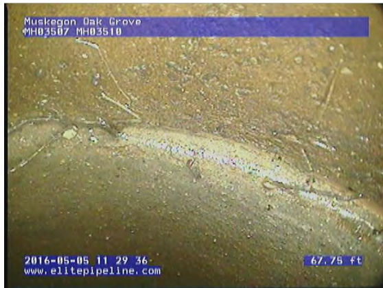
GM3676_29b5a4f6-782c-44a4-b604-e6dda5d2d56c_20160505_113112_729.jpg, 00:09:59, 67.07 Roots Fine Joint from 10 o'clock to 11 o'clock, within 8 inch
