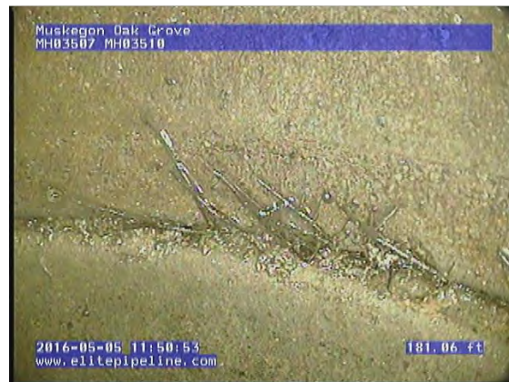
GM3676_29b5a4f6-782c-44a4-b604-e6dda5d2d56c_20160505_115230_357.jpg, 00:25:05, 179.99 Roots Fine Joint from 9 o'clock to 1 o'clock, within 8 inch
