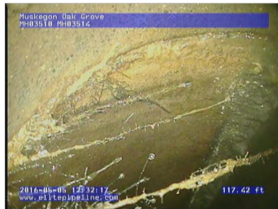
GM3683_ed2824f5-d3e3-4757-88d6-d4208adc31ee_20160505_123354_156.jpg, 00:12:29, 116.49 Infiltration Dripper from 12 o'clock to 3 o'clock, within 8 inch
