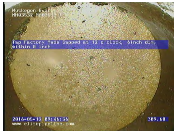
GM3701_62c62d3f-fa26-4182-aa9d-10e119c32db3_20160512_094815_242.jpg, 00:22:07, 308.55 Tap Factory Made Capped at 12 o'clock, 6inch dim, within 8 inch
