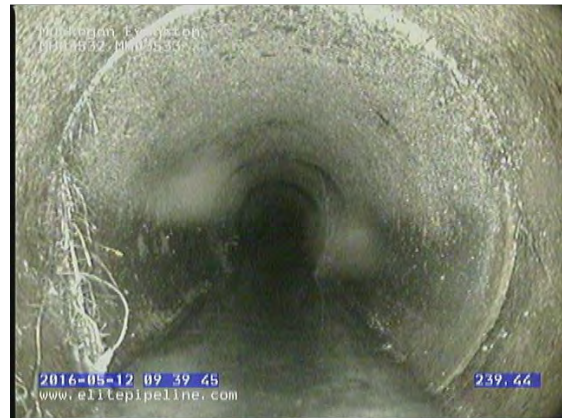
GM3701_62c62d3f-fa26-4182-aa9d-10e119c32db3_20160512_094104_451.jpg, 00:16:08, 239.43 Roots Fine Joint from 7 o'clock to 10 o'clock, within 8 inch
