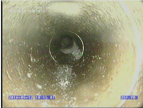
GM3702_bffedebf-8262-4dd8-8638-19abd94e99a5_20160512_101620_298.jpg, 00:20:50, 250.29 Tap Break-In at 12 o'clock, 6inch dim, within 8 inch
