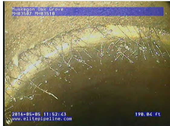
GM3676_29b5a4f6-782c-44a4-b604-e6dda5d2d56c_20160505_115419_978.jpg, 00:26:29, 189.32 Roots Fine Joint from 8 o'clock to 2 o'clock, within 8 inch
