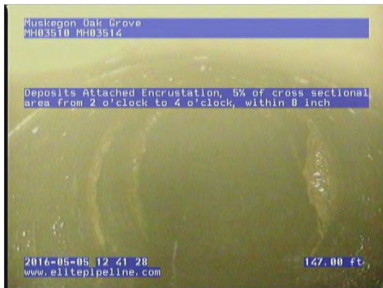
GM3683_ed2824f5-d3e3-4757-88d6-d4208adc31ee_20160505_124305_614.jpg, 00:18:33, 147.00 Deposits Attached Encrustation, 5% of cross sectional area from 2 o'clock to 4 o'clock, within 8 inch
