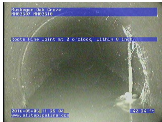
GM3676_29b5a4f6-782c-44a4-b604-e6dda5d2d56c_20160505_112641_393.jpg, 00:06:26, 42.24 Roots Fine Joint at 2 o'clock, within 8 inch
