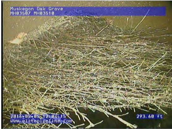
GM3676_29b5a4f6-782c-44a4-b604-e6dda5d2d56c_20160505_120552_145.jpg, 00:36:28, 292.77 Roots Ball Joint from 7 o'clock to 5 o'clock, 75% lost, within 8 inch
