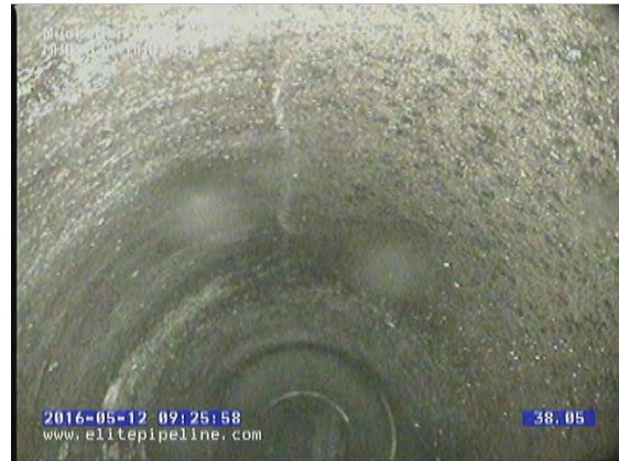
GM3701_62c62d3f-fa26-4182-aa9d-10e119c32db3_20160512_092717_543.jpg, 00:03:15, 38.04 Crack Longitudinal at 12 o'clock, within 8 inch
