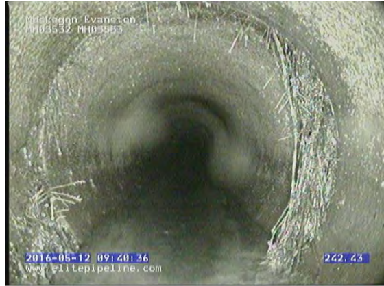
GM3701_62c62d3f-fa26-4182-aa9d-10e119c32db3_20160512_094155_139.jpg, 00:16:44, 242.41 Roots Fine Joint from 7 o'clock to 5 o'clock, within 8 inch
