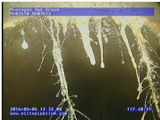
GM3683_ed2824f5-d3e3-4757-88d6-d4208adc31ee_20160505_123345_591.jpg, 00:12:29, 116.49 Infiltration Dripper from 12 o'clock to 3 o'clock, within 8 inch
