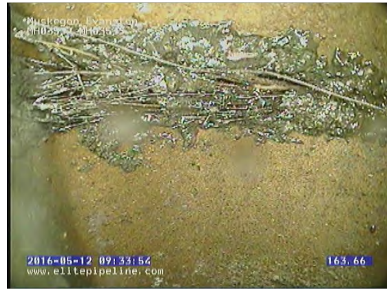
GM3701_62c62d3f-fa26-4182-aa9d-10e119c32db3_20160512_093513_265.jpg, 00:10:35, 162.52 Roots Fine Joint from 7 o'clock to 5 o'clock, within 8 inch
