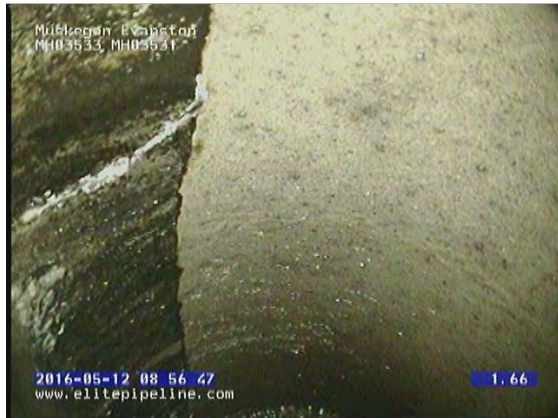
GM3700_d760bc2d-7738-420b-a21c-0e3d9fae79d8_20160512_085806_617.jpg, 00:02:31, 1.66 Infiltration Runner at 9 o'clock, within 8 inch
