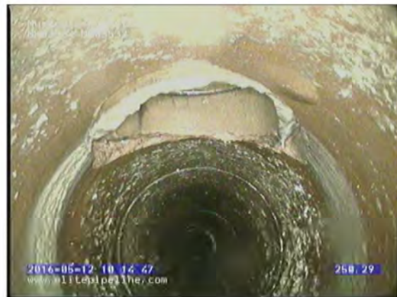
GM3702_bffedebf-8262-4dd8-8638-19abd94e99a5_20160512_101606_075.jpg, 00:20:50, 250.29 Tap Break-In at 12 o'clock, 6inch dim, within 8 inch
