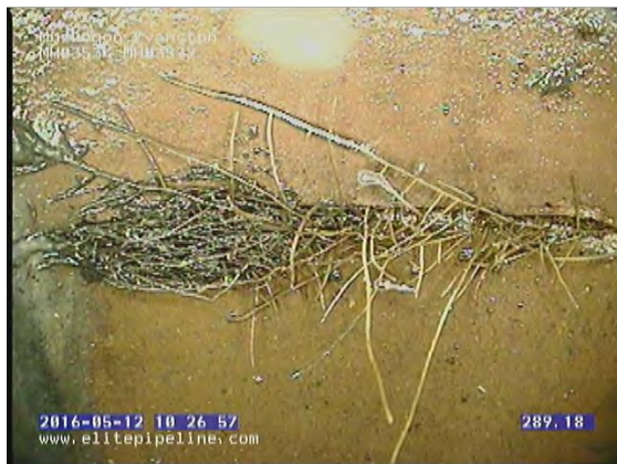
GM3702_bffedebf-8262-4dd8-8638-19abd94e99a5_20160512_102815_939.jpg, 00:26:54, 288.13 Roots Fine Joint from 7 o'clock to 10 o'clock, within 8 inch
