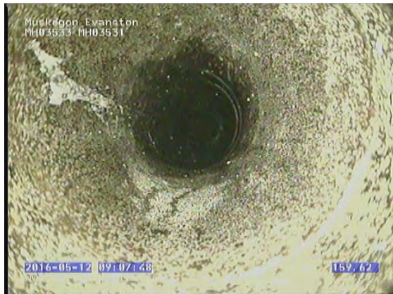
GM3700_d760bc2d-7738-420b-a21c-0e3d9fae79d8_20160512_090907_178.jpg, 00:11:02, 158.48 Tap Factory Made at 12 o'clock, 6inch dim, within 8 inch
