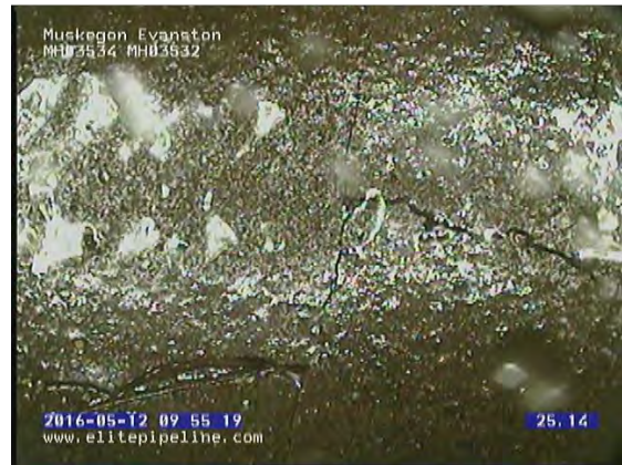
GM3702_bffedebf-8262-4dd8-8638-19abd94e99a5_20160512_095638_538.jpg, 00:02:55, 24.98 Crack Multiple from 11 o'clock to 1 o'clock, within 8 inch
