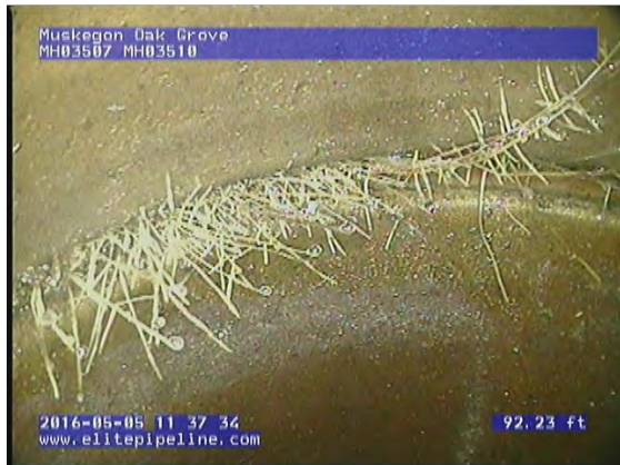
GM3676_29b5a4f6-782c-44a4-b604-e6dda5d2d56c_20160505_113911_158.jpg, 00:14:23, 91.19 Roots Fine Joint from 9 o'clock to 5 o'clock, Start, within 8 inch
