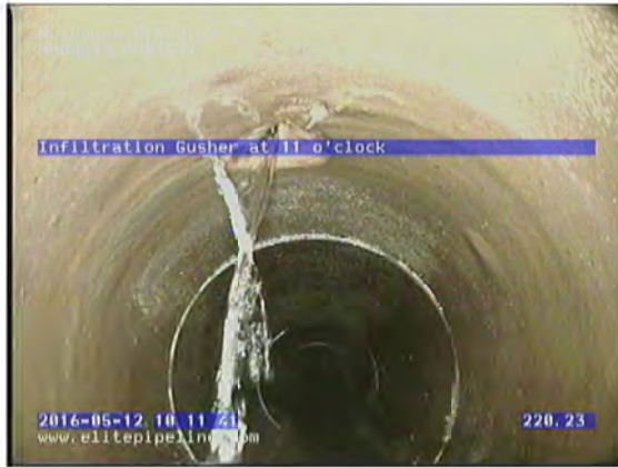
GM3702_bffedebf-8262-4dd8-8638-19abd94e99a5_20160512_101259_971.jpg, 00:18:07, 220.23 Infiltration Gusher at 11 o'clock
