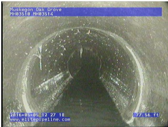
GM3683_ed2824f5-d3e3-4757-88d6-d4208adc31ee_20160505_122855_232.jpg, 00:08:34, 77.56 Roots Fine Joint from 9 o'clock to 11 o'clock, within 8 inch
