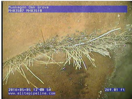
GM3676_29b5a4f6-782c-44a4-b604-e6dda5d2d56c_20160505_120227_569.jpg, 00:33:56, 268.17 Roots Fine Joint from 3 o'clock to 5 o'clock, within 8 inch
