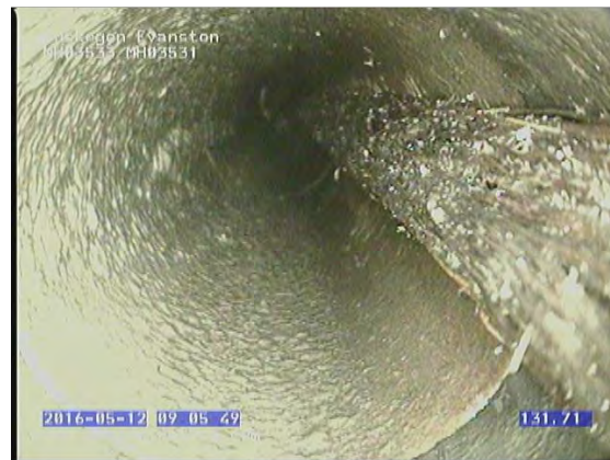
GM3700_d760bc2d-7738-420b-a21c-0e3d9fae79d8_20160512_090708_018.jpg, 00:09:15, 130.36 Tap Factory Made at 12 o'clock, 6inch dim, within 8 inch
