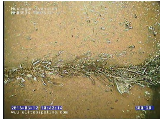
GM3702_bffedebf-8262-4dd8-8638-19abd94e99a5_20160512_104332_914.jpg, 00:38:38, 379.58 Roots Fine Joint from 2 o'clock to 4 o'clock, within 8 inch
