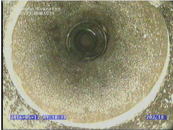
GM3700_d760bc2d-7738-420b-a21c-0e3d9fae79d8_20160512_091136_847.jpg, 00:13:23, 200.60 Tap Factory Made at 12 o'clock, 6inch dim, within 8 inch
