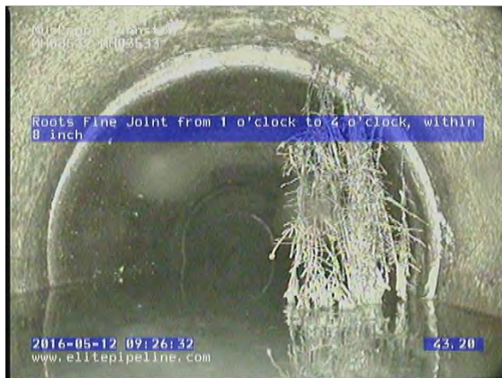
GM3701_62c62d3f-fa26-4182-aa9d-10e119c32db3_20160512_092751_813.jpg, 00:03:45, 43.20 Roots Fine Joint from 1 o'clock to 4 o'clock, within 8 inch
