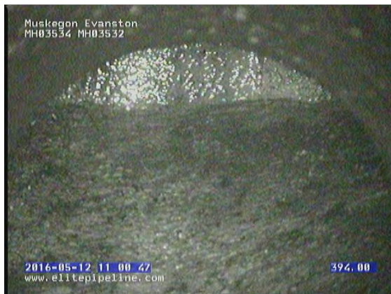
GM3702_bffedebf-8262-4dd8-8638-19abd94e99a5_20160512_110206_027.jpg, 00:39:52, 394.00 Manhole, upstream, survey complete. possibly to MH02761
