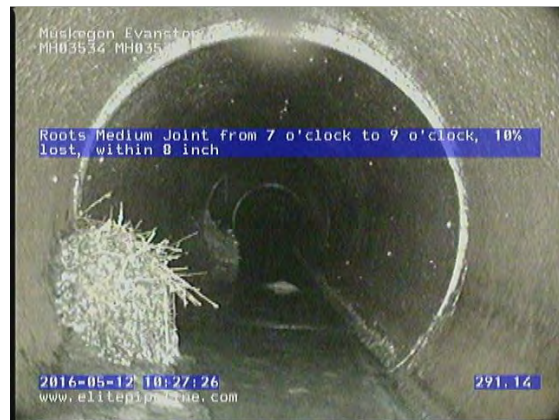
GM3702_bffedebf-8262-4dd8-8638-19abd94e99a5_20160512_102845_351.jpg, 00:27:24, 291.13 Roots Medium Joint from 7 o'clock to 9 o'clock, 10% lost, within 8 inch
