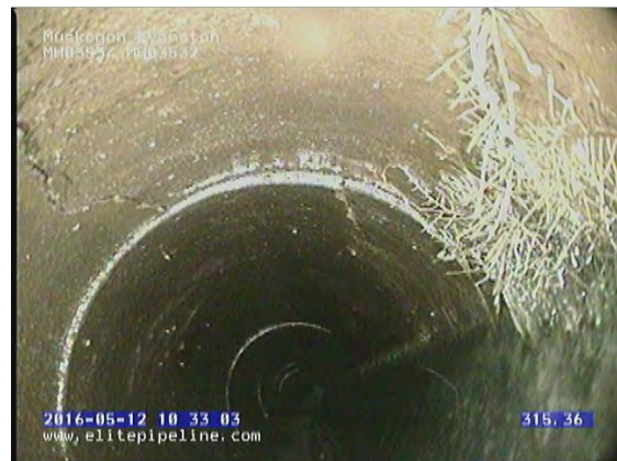
GM3702_bffedebf-8262-4dd8-8638-19abd94e99a5_20160512_103422_133.jpg, 00:31:47, 315.36 Crack Spiral from 2 o'clock to 4 o'clock, within 8 inch
