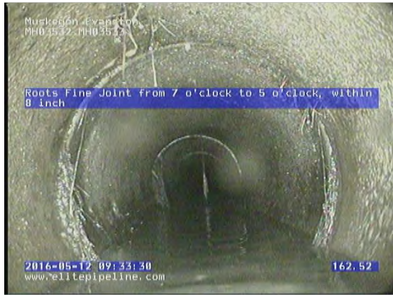
GM3701_62c62d3f-fa26-4182-aa9d-10e119c32db3_20160512_093449_767.jpg, 00:10:35, 162.52 Roots Fine Joint from 7 o'clock to 5 o'clock, within 8 inch
