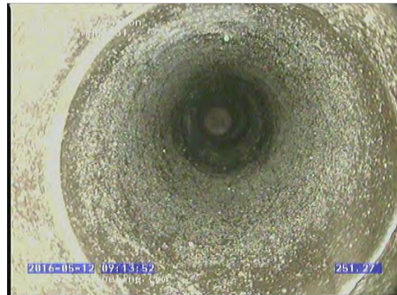
GM3700_d760bc2d-7738-420b-a21c-0e3d9fae79d8_20160512_091511_684.jpg, 00:16:30, 250.29 Tap Factory Made at 12 o'clock, 6inch dim, within 8 inch
