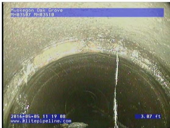
GM3676_29b5a4f6-782c-44a4-b604-e6dda5d2d56c_20160505_112044_947.jpg, 00:01:33, 2.57 Infiltration Gusher from 10 o'clock to 1 o'clock, within 8 inch
