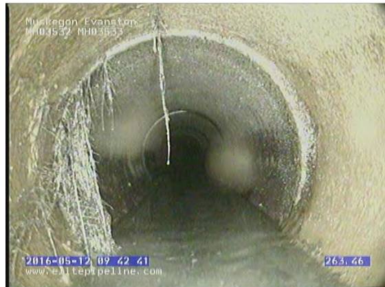
GM3701_62c62d3f-fa26-4182-aa9d-10e119c32db3_20160512_094400_230.jpg, 00:18:40, 263.46 Roots Fine Joint from 7 o'clock to 12 o'clock, within 8 inch
