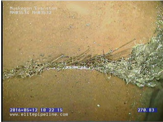
GM3702_bffedebf-8262-4dd8-8638-19abd94e99a5_20160512_102333_883.jpg, 00:23:57, 270.04 Roots Fine Joint from 10 o'clock to 5 o'clock, within 8 inch
