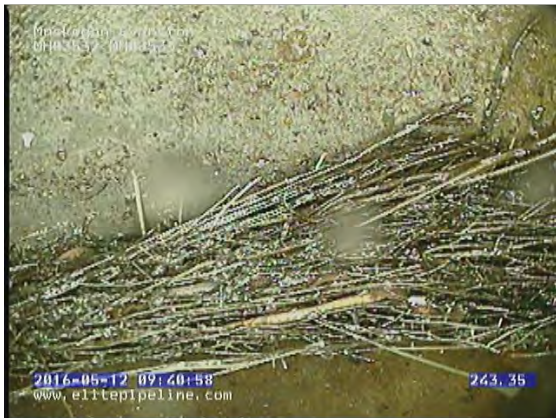
GM3701_62c62d3f-fa26-4182-aa9d-10e119c32db3_20160512_094217_264.jpg, 00:16:44, 242.41 Roots Fine Joint from 7 o'clock to 5 o'clock, within 8 inch
