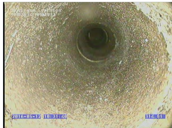
GM3702_bffedebf-8262-4dd8-8638-19abd94e99a5_20160512_103258_925.jpg, 00:30:29, 313.46 Tap Break-In at 12 o'clock, 6inch dim
