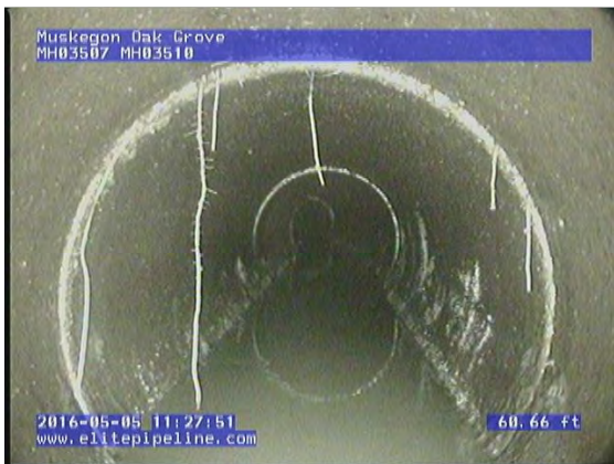
GM3676_29b5a4f6-782c-44a4-b604-e6dda5d2d56c_20160505_112928_428.jpg, 00:08:41, 60.65 Roots Fine Joint from 9 o'clock to 2 o'clock, within 8 inch
