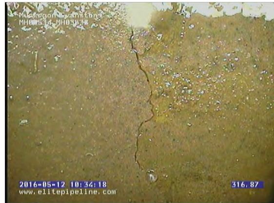
GM3702_bffedebf-8262-4dd8-8638-19abd94e99a5_20160512_103537_751.jpg, 00:32:39, 316.87 Crack Longitudinal at 3 o'clock, within 8 inch
