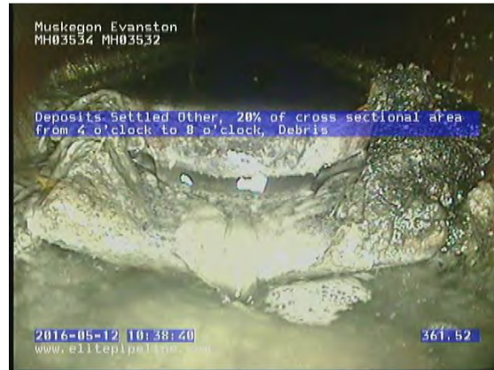
GM3702_bffedebf-8262-4dd8-8638-19abd94e99a5_20160512_103959_750.jpg, 00:36:32, 361.52 Deposits Settled Other, 20% of cross sectional area from 4 o'clock to 8 o'clock, Debris
