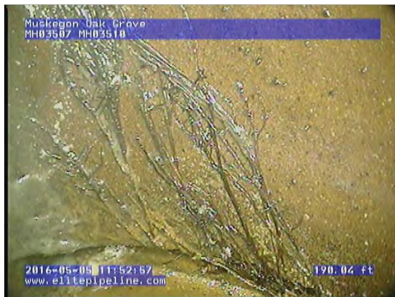
GM3676_29b5a4f6-782c-44a4-b604-e6dda5d2d56c_20160505_115434_520.jpg, 00:26:29, 189.32 Roots Fine Joint from 8 o'clock to 2 o'clock, within 8 inch
