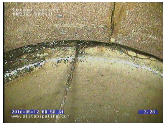
GM3700_d760bc2d-7738-420b-a21c-0e3d9fae79d8_20160512_090010_169.jpg, 00:03:29, 2.89 Roots Fine Joint at 12 o'clock, within 8 inch
