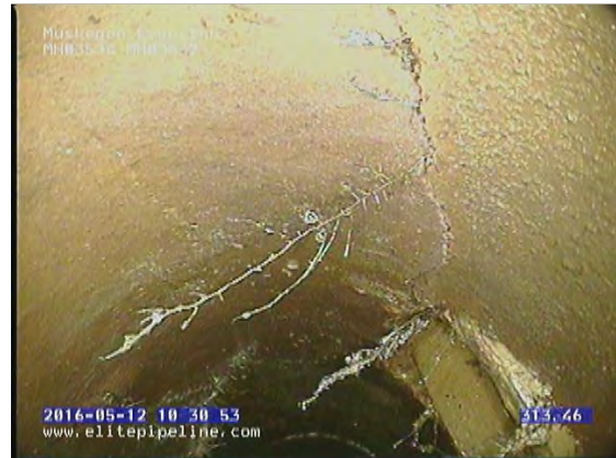
GM3702_bffedebf-8262-4dd8-8638-19abd94e99a5_20160512_103212_158.jpg, 00:30:07, 313.46 Roots Fine Barrell at 10 o'clock, within 8 inch
