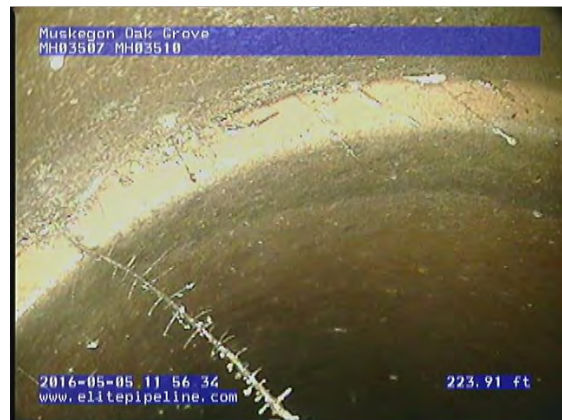
GM3676_29b5a4f6-782c-44a4-b604-e6dda5d2d56c_20160505_115810_782.jpg, 00:29:53, 223.07 Roots Fine Joint from 10 o'clock to 2 o'clock, within 8 inch
