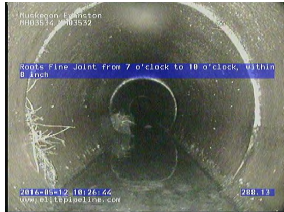
GM3702_bffedebf-8262-4dd8-8638-19abd94e99a5_20160512_102803_564.jpg, 00:26:54, 288.13 Roots Fine Joint from 7 o'clock to 10 o'clock, within 8 inch
