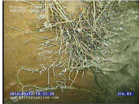
GM3702_bffedebf-8262-4dd8-8638-19abd94e99a5_20160512_103447_553.jpg, 00:31:58, 315.36 Roots Fine Barrell at 4 o'clock, within 8 inch
