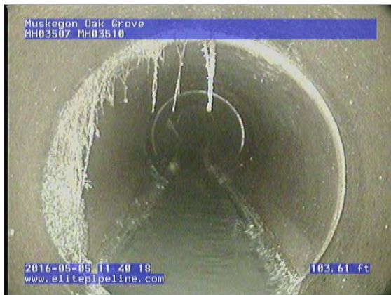
GM3676_29b5a4f6-782c-44a4-b604-e6dda5d2d56c_20160505_114154_834.jpg, 00:16:53, 103.61 Roots Medium Joint from 7 o'clock to 12 o'clock, 5% lost, within 8 inch
