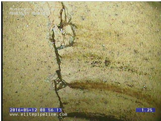
GM3700_d760bc2d-7738-420b-a21c-0e3d9fae79d8_20160512_085732_800.jpg, 00:01:23, 1.00 Crack Multiple from 12 o'clock to 12 o'clock, within 8 inch
