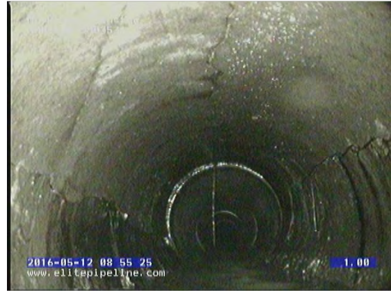
GM3700_d760bc2d-7738-420b-a21c-0e3d9fae79d8_20160512_085644_396.jpg, 00:01:23, 1.00 Crack Multiple from 12 o'clock to 12 o'clock, within 8 inch
