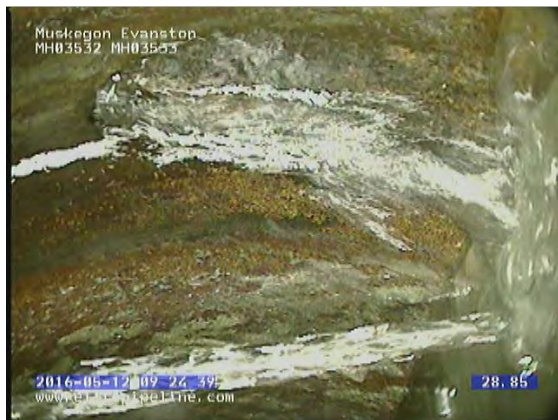
GM3701_62c62d3f-fa26-4182-aa9d-10e119c32db3_20160512_092558_697.jpg, 00:01:55, 27.89 Infiltration Gusher from 12 o'clock to 4 o'clock, within 8 inch
