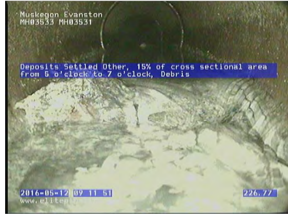
GM3700_d760bc2d-7738-420b-a21c-0e3d9fae79d8_20160512_091310_103.jpg, 00:14:59, 226.77 Deposits Settled Other, 15% of cross sectional area from 5 o'clock to 7 o'clock, Debris
