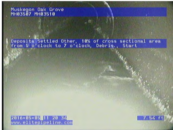
GM3676_29b5a4f6-782c-44a4-b604-e6dda5d2d56c_20160505_112211_171.jpg, 00:02:46, 7.54 Deposits Settled Other, 10% of cross sectional area from 5 o'clock to 7 o'clock, Debris., Start
