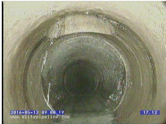
GM3700_d760bc2d-7738-420b-a21c-0e3d9fae79d8_20160512_090138_517.jpg, 00:03:48, 16.89 Tap Factory Made Active at 12 o'clock, 6inch dim, within 8 inch
