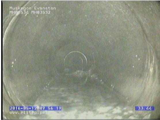
GM3702_bffedebf-8262-4dd8-8638-19abd94e99a5_20160512_095737_885.jpg, 00:03:59, 33.44 Infiltration Runner at 2 o'clock, within 8 inch
