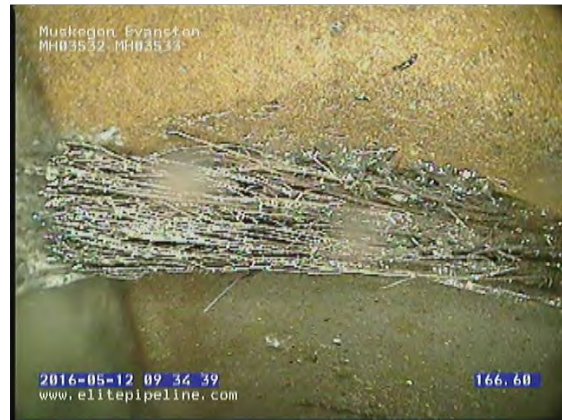
GM3701_62c62d3f-fa26-4182-aa9d-10e119c32db3_20160512_093558_113.jpg, 00:11:17, 165.85 Roots Fine Joint from 7 o'clock to 1 o'clock, within 8 inch
