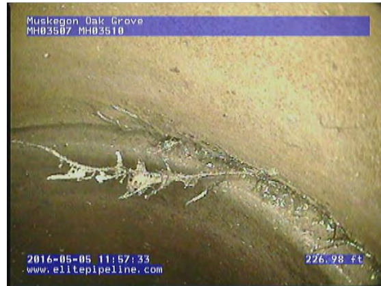
GM3676_29b5a4f6-782c-44a4-b604-e6dda5d2d56c_20160505_115909_956.jpg, 00:30:43, 226.34 Roots Fine Joint from 9 o'clock to 12 o'clock, within 8 inch
