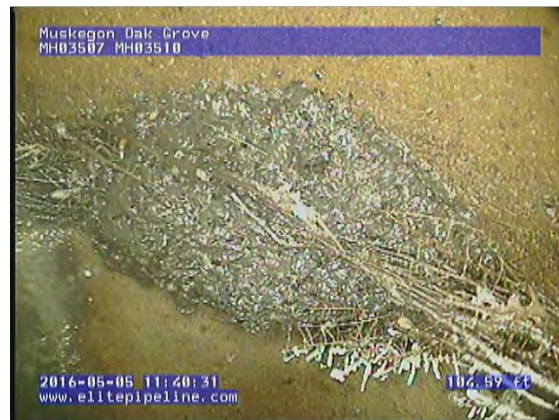
GM3676_29b5a4f6-782c-44a4-b604-e6dda5d2d56c_20160505_114208_439.jpg, 00:16:53, 103.61 Roots Medium Joint from 7 o'clock to 12 o'clock, 5% lost, within 8 inch
