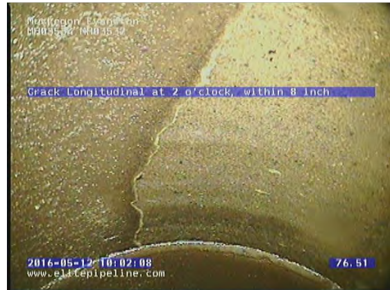
GM3702_bffedebf-8262-4dd8-8638-19abd94e99a5_20160512_100327_338.jpg, 00:08:52, 76.51 Crack Longitudinal at 2 o'clock, within 8 inch
