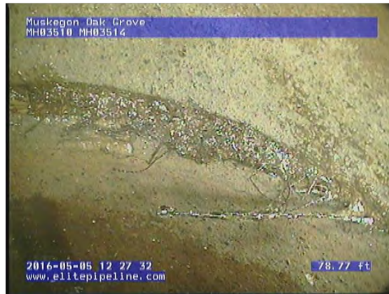
GM3683_ed2824f5-d3e3-4757-88d6-d4208adc31ee_20160505_122908_817.jpg, 00:08:34, 77.56 Roots Fine Joint from 9 o'clock to 11 o'clock, within 8 inch
