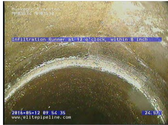
GM3702_bffedebf-8262-4dd8-8638-19abd94e99a5_20160512_095554_304.jpg, 00:02:33, 24.56 Infiltration Runner at 12 o'clock, within 8 inch
