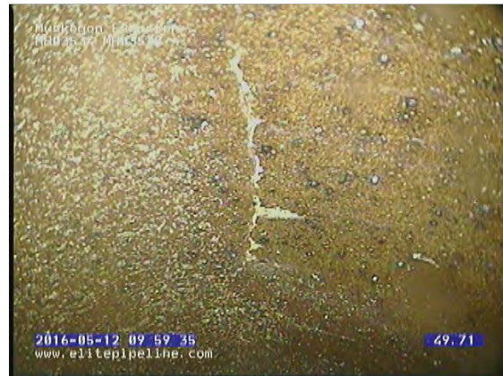
GM3702_bffedebf-8262-4dd8-8638-19abd94e99a5_20160512_100054_862.jpg, 00:06:32, 49.70 Crack Longitudinal at 2 o'clock, within 8 inch
