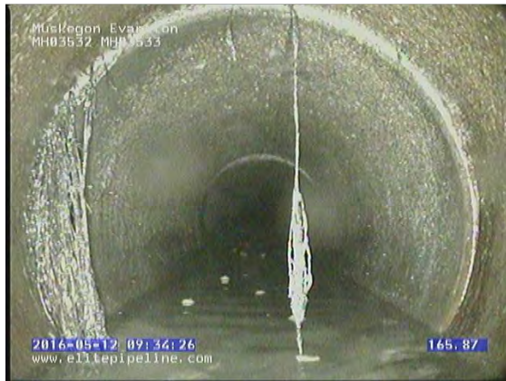
GM3701_62c62d3f-fa26-4182-aa9d-10e119c32db3_20160512_093545_250.jpg, 00:11:17, 165.85 Roots Fine Joint from 7 o'clock to 1 o'clock, within 8 inch
