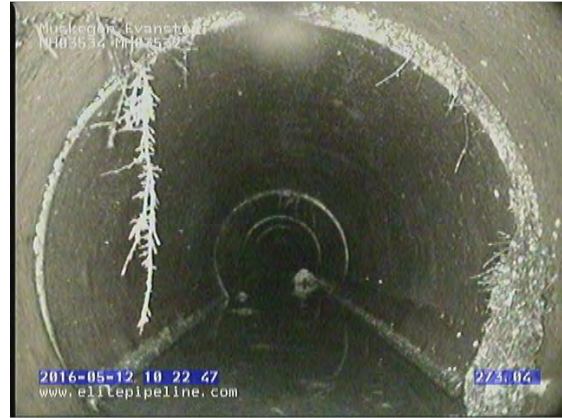
GM3702_bffedebf-8262-4dd8-8638-19abd94e99a5_20160512_102406_541.jpg, 00:24:38, 273.04 Roots Fine Joint from 10 o'clock to 5 o'clock, within 8 inch
