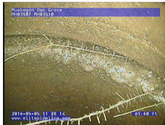
GM3676_29b5a4f6-782c-44a4-b604-e6dda5d2d56c_20160505_112951_415.jpg, 00:08:41, 60.65 Roots Fine Joint from 9 o'clock to 2 o'clock, within 8 inch
