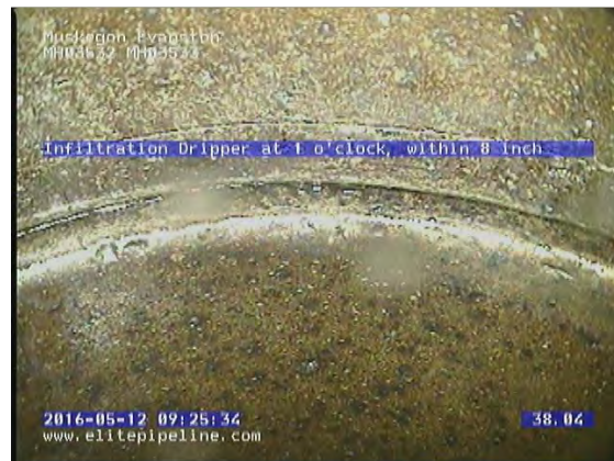
GM3701_62c62d3f-fa26-4182-aa9d-10e119c32db3_20160512_092653_465.jpg, 00:03:02, 38.04 Infiltration Dripper at 1 o'clock, within 8 inch
