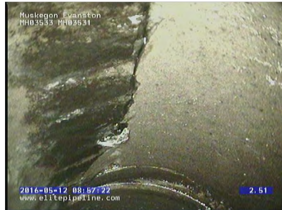
GM3700_d760bc2d-7738-420b-a21c-0e3d9fae79d8_20160512_085841_800.jpg, 00:02:31, 1.66 Infiltration Runner at 9 o'clock, within 8 inch
