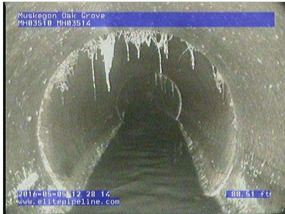
GM3683_ed2824f5-d3e3-4757-88d6-d4208adc31ee_20160505_122951_580.jpg, 00:09:18, 80.51 Roots Fine Joint from 7 o'clock to 5 o'clock, Start, within 8 inch
