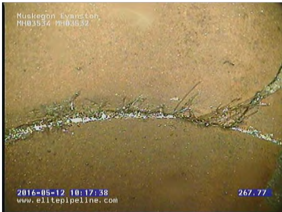
GM3702_bffedebf-8262-4dd8-8638-19abd94e99a5_20160512_101856_978.jpg, 00:23:16, 267.77 Roots Fine Joint from 2 o'clock to 4 o'clock, within 8 inch
