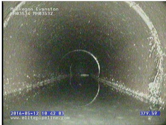
GM3702_bffedebf-8262-4dd8-8638-19abd94e99a5_20160512_104322_053.jpg, 00:38:38, 379.58 Roots Fine Joint from 2 o'clock to 4 o'clock, within 8 inch
