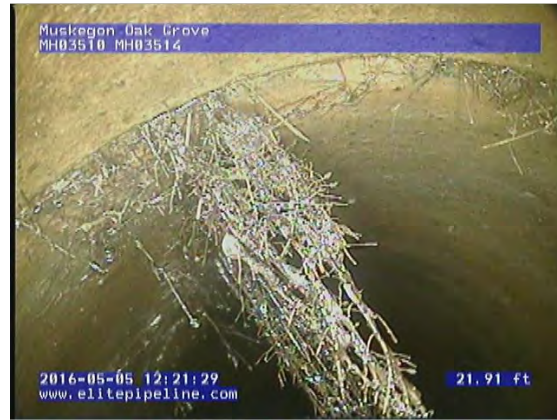
GM3683_ed2824f5-d3e3-4757-88d6-d4208adc31ee_20160505_122306_316.jpg, 00:03:10, 20.89 Roots Fine Joint from 10 o'clock to 3 o'clock, within 8 inch
