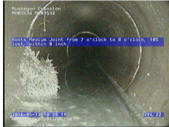
GM3702_bffedebf-8262-4dd8-8638-19abd94e99a5_20160512_102938_445.jpg, 00:27:58, 294.21 Roots Medium Joint from 7 o'clock to 8 o'clock, 10% lost, within 8 inch
