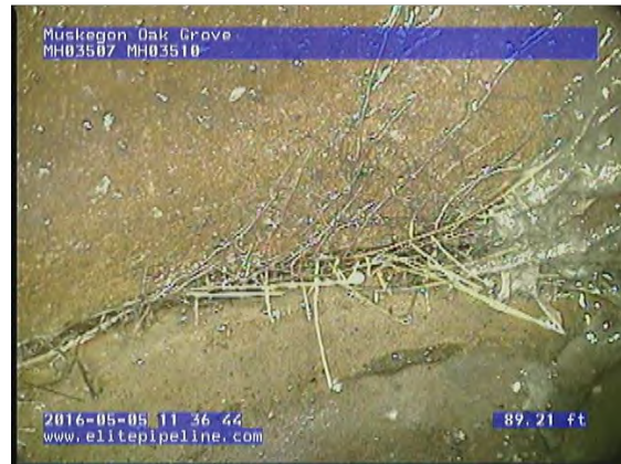
GM3676_29b5a4f6-782c-44a4-b604-e6dda5d2d56c_20160505_113821_665.jpg, 00:13:13, 87.89 Roots Fine Joint from 9 o'clock to 5 o'clock, within 8 inch
