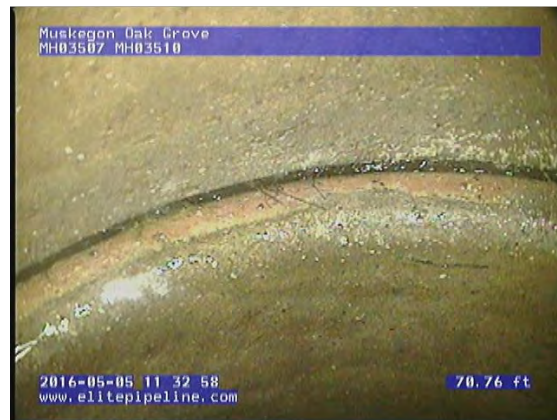
GM3676_29b5a4f6-782c-44a4-b604-e6dda5d2d56c_20160505_113435_339.jpg, 00:11:13, 70.76 Roots Fine Joint from 9 o'clock to 3 o'clock, within 8 inch
