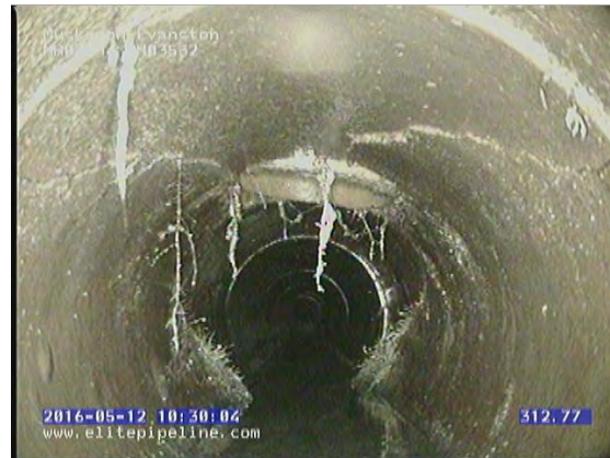
GM3702_bffedebf-8262-4dd8-8638-19abd94e99a5_20160512_103123_004.jpg, 00:29:31, 312.77 Crack Multiple from 10 o'clock to 2 o'clock, within 8 inch
