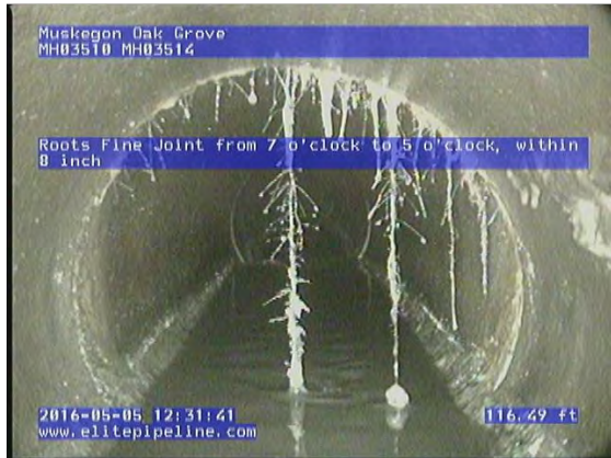
GM3683_ed2824f5-d3e3-4757-88d6-d4208adc31ee_20160505_123317_777.jpg, 00:12:18, 116.49 Roots Fine Joint from 7 o'clock to 5 o'clock, within 8 inch
