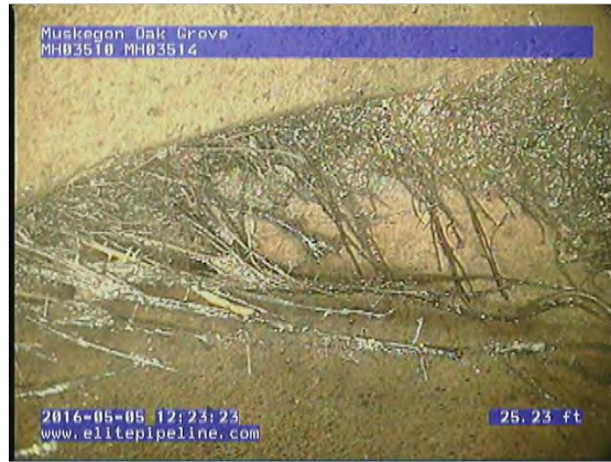
GM3683_ed2824f5-d3e3-4757-88d6-d4208adc31ee_20160505_122500_362.jpg, 00:04:49, 24.44 Roots Fine Joint from 10 o'clock to 4 o'clock, within 8 inch
