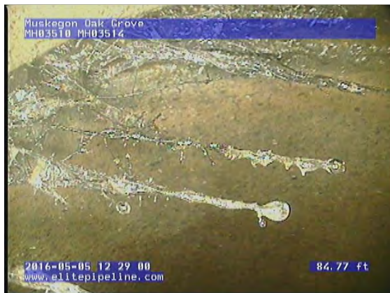
GM3683_ed2824f5-d3e3-4757-88d6-d4208adc31ee_20160505_123037_540.jpg, 00:09:44, 83.98 Infiltration Dripper at 2 o'clock, within 8 inch
