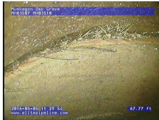
GM3676_29b5a4f6-782c-44a4-b604-e6dda5d2d56c_20160505_113131_305.jpg, 00:09:59, 67.07 Roots Fine Joint from 10 o'clock to 11 o'clock, within 8 inch
