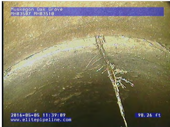
GM3676_29b5a4f6-782c-44a4-b604-e6dda5d2d56c_20160505_114046_033.jpg, 00:15:51, 97.59 Infiltration Dripper at 12 o'clock, within 8 inch
