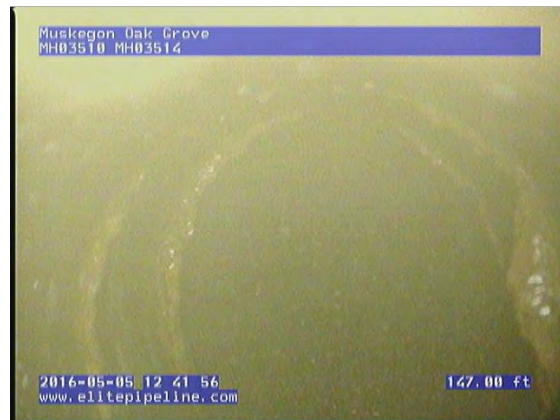
GM3683_ed2824f5-d3e3-4757-88d6-d4208adc31ee_20160505_124332_935.jpg, 00:18:48, 147.00 Infiltration Dripper from 11 o'clock to 12 o'clock, within 8 inch
