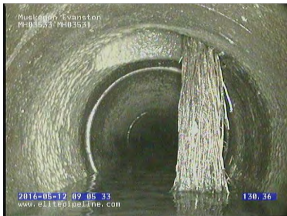
GM3700_d760bc2d-7738-420b-a21c-0e3d9fae79d8_20160512_090652_594.jpg, 00:09:15, 130.36 Tap Factory Made at 12 o'clock, 6inch dim, within 8 inch
