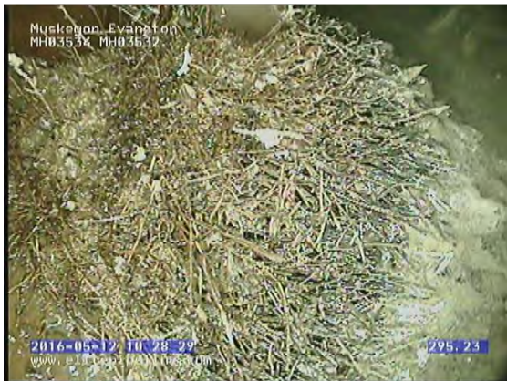
GM3702_bffedebf-8262-4dd8-8638-19abd94e99a5_20160512_102948_077.jpg, 00:27:58, 294.21 Roots Medium Joint from 7 o'clock to 8 o'clock, 10% lost, within 8 inch
