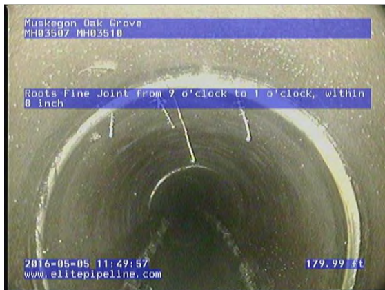
GM3676_29b5a4f6-782c-44a4-b604-e6dda5d2d56c_20160505_115133_828.jpg, 00:25:05, 179.99 Roots Fine Joint from 9 o'clock to 1 o'clock, within 8 inch
