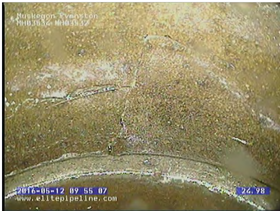
GM3702_bffedebf-8262-4dd8-8638-19abd94e99a5_20160512_095626_606.jpg, 00:02:33, 24.56 Infiltration Runner at 12 o'clock, within 8 inch
