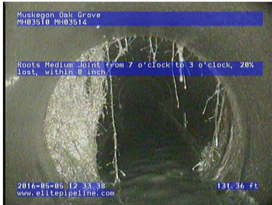
GM3683_ed2824f5-d3e3-4757-88d6-d4208adc31ee_20160505_123514_953.jpg, 00:13:49, 131.34 Roots Medium Joint from 7 o'clock to 3 o'clock, 20% lost, within 8 inch
