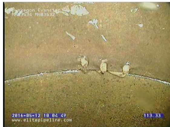
GM3702_bffedebf-8262-4dd8-8638-19abd94e99a5_20160512_100607_953.jpg, 00:11:13, 112.19 Infiltration Runner at 11 o'clock, within 8 inch
