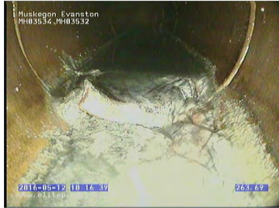
GM3702_bffedebf-8262-4dd8-8638-19abd94e99a5_20160512_101758_240.jpg, 00:22:18, 263.69 Deposits Settled Other, 5% of cross sectional area from 5 o'clock to 7 o'clock, within 8 inch, Debris
