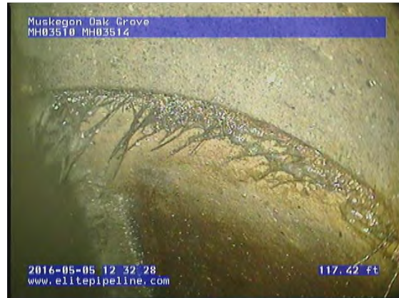
GM3683_ed2824f5-d3e3-4757-88d6-d4208adc31ee_20160505_123405_642.jpg, 00:12:18, 116.49 Roots Fine Joint from 7 o'clock to 5 o'clock, within 8 inch
